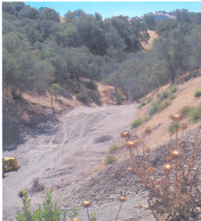
Photo No. 2 Fill Material Placed in Canyon at the Site (Looking Downstream)
